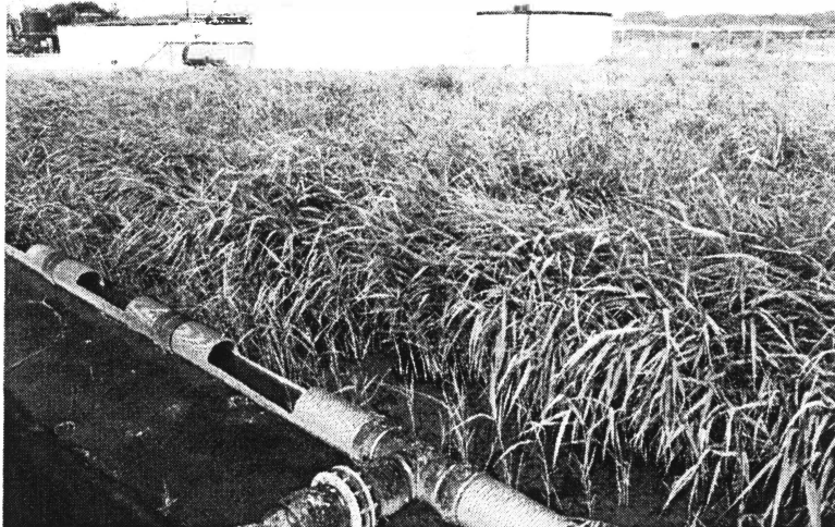
Figure 3. Efford Leachate Treatment Plant, view from the reed bed, 10 July 2003.
