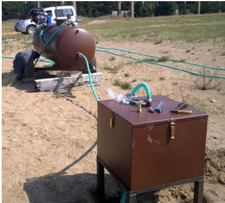
Figure 3. Pump-and-treat system using carbon powder cassettes (in the box).
