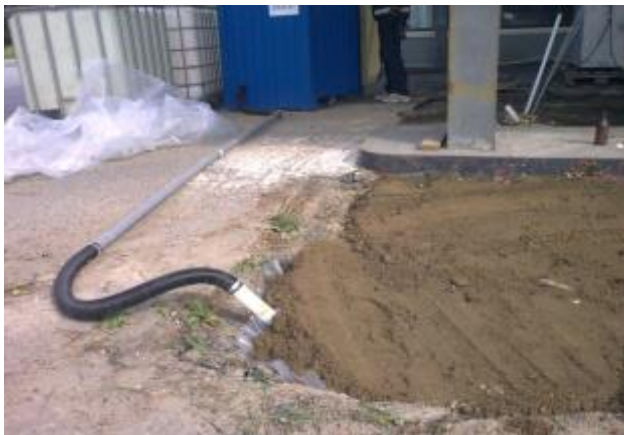
Figure 2: Perforated tubing was installed into the electro-kinetically dried gasoline contaminated soil. The tubing was connected to a vacuum pump and active charcoal to collect the gasoline.
