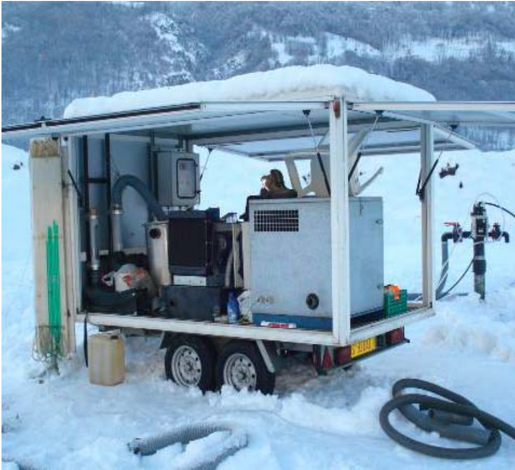
Figure 5. The air injection/gas extraction mobile unit used for the tests
